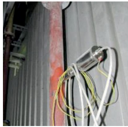
Adsorber / flue gas cleaning
